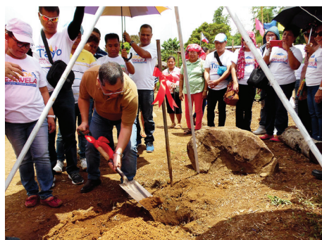
Mayor Yulo leads the groundbreaking of the Najaba Elementary School- Tabucol Extension at Barangay Bacong in the presence of DepEd officials led by Dr. Ma. Lorlinie Ortillo and school teachers.
